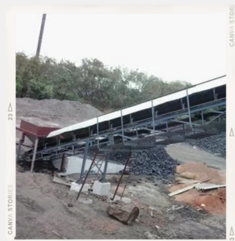
MATERIAL HANDLING SYSTEM
