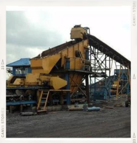
COAL HANDLING PLANT
